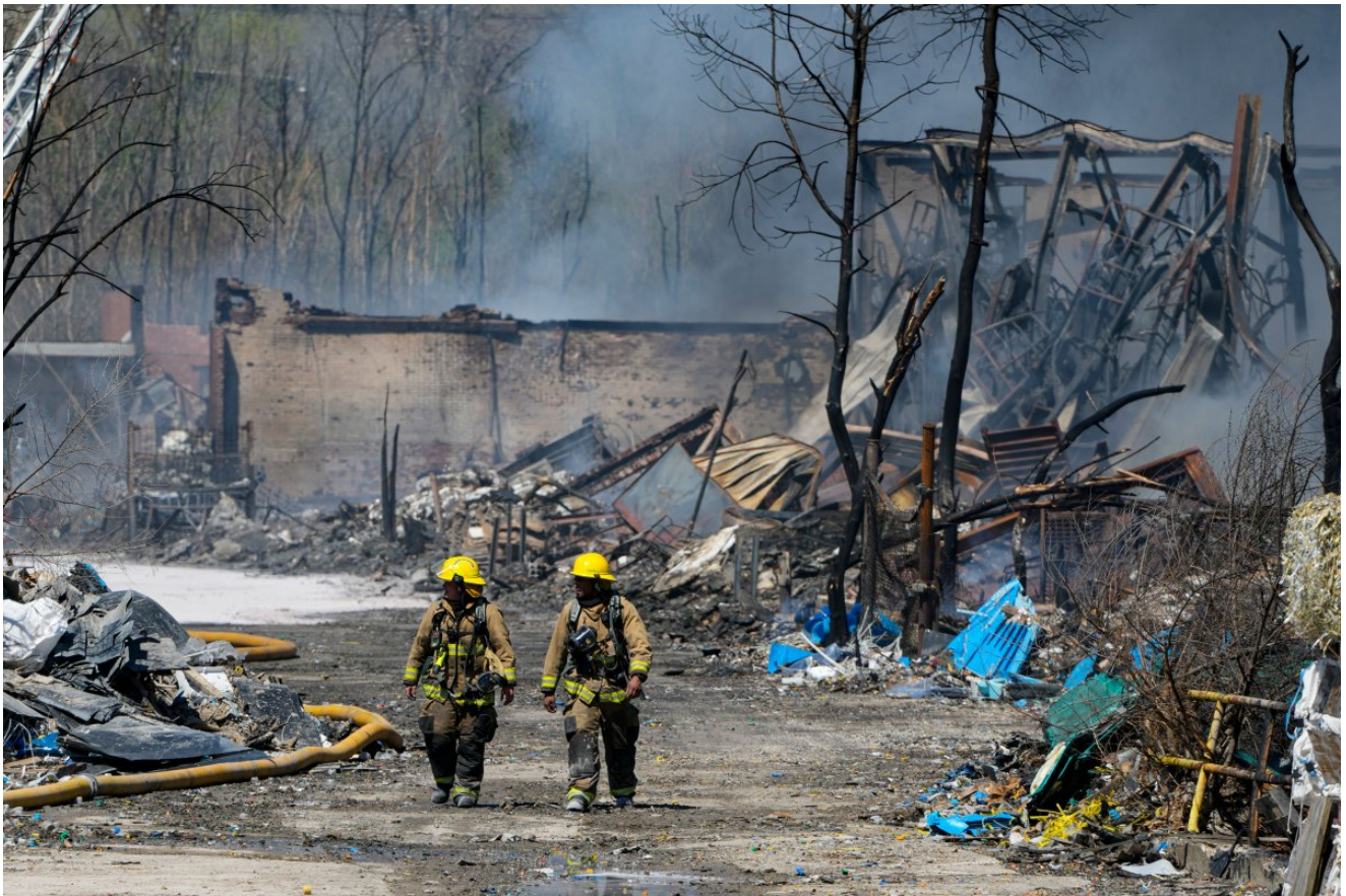
Firefighters walk out of the site of an industrial fire in Richmond, Ind., on April 12, 2023.
