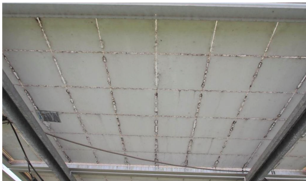
FIGURE 2 Full polyamide backsheet showing cracks after several years of outdoor operation [Colour figure can be viewed at wileyonlinelibrary.com ]
